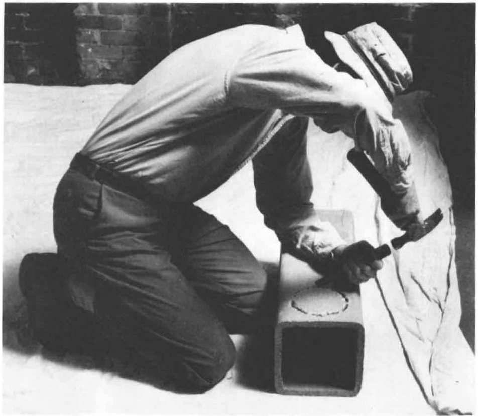
The first section of liner is cut to receive the thimble fitting, a tricky business since the ceramic material is very brittle. Closely spaced holes are first drilled along the cut-line; then the waste piece is knocked out with a hammer and chisel, as shown.
